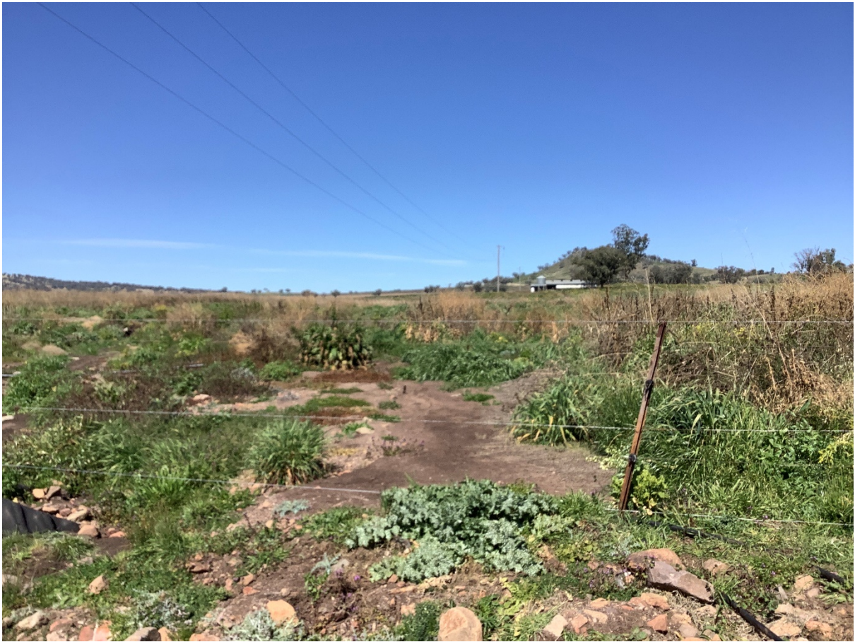
Plate 1 Facing south from northern end of project area showing erosion along drainage line.
